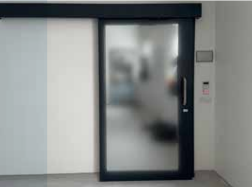
▲ Bosnia - Dobo: Operating Block, Simple Sealing Doors
